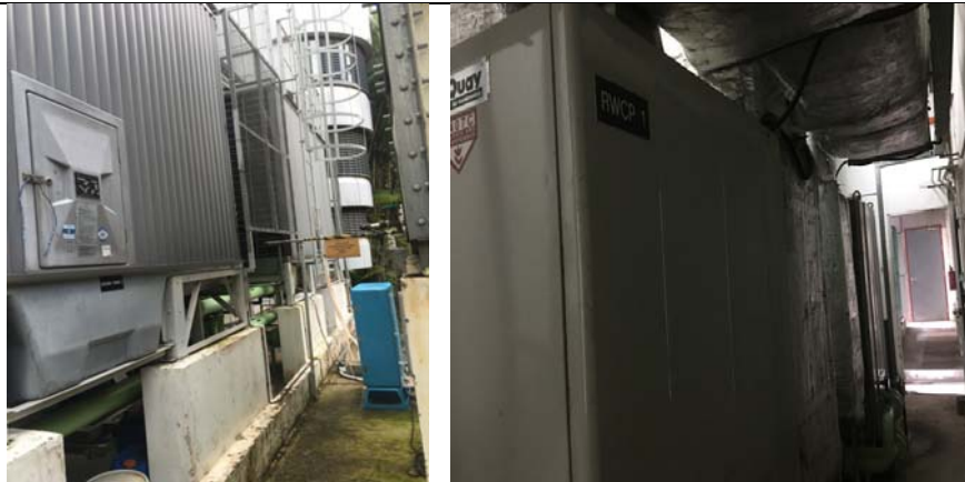
Figure 2. Valley Block CT1 & CT2 with DCI installation and RWCP1 & RWCP2
