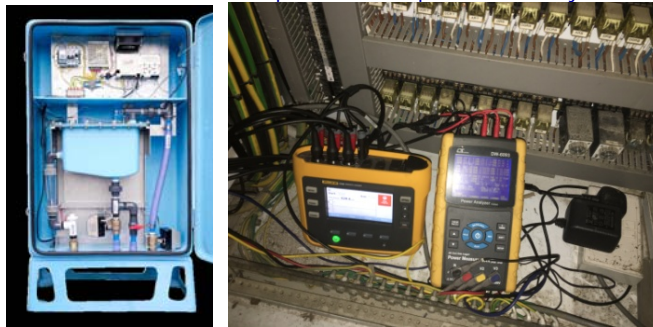
Figure 3. DCI system and portable power meters
